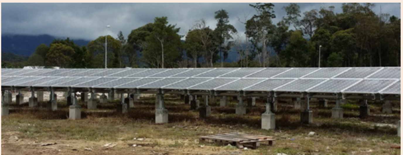
Solar farm for rural electrification programme in Bario.
