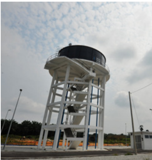
An elevated water tank under Program Bekalan Air Luar Bandar.
